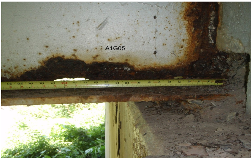
Figure 3.1: Presents a Typical Location of Uniform Corrosion on a Composite Steel Girder Bridge. The Picture is Courtesy of The Nebraska Department Of Roads.
